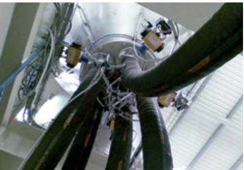
Micro-silica conveying 1 silo feeds 5 separate lines.
