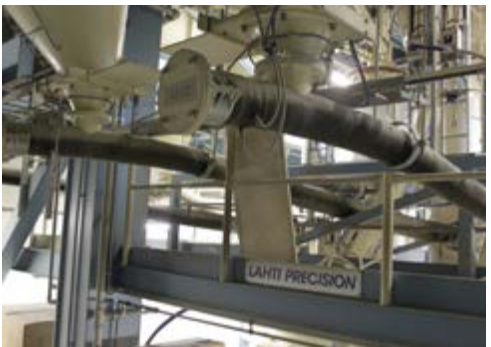
Cement dosing application
